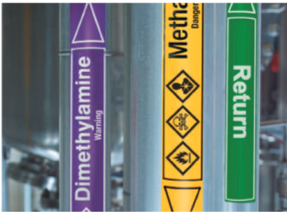
Pipe & valve marking
