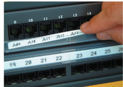
Punch block & patch panel labels
